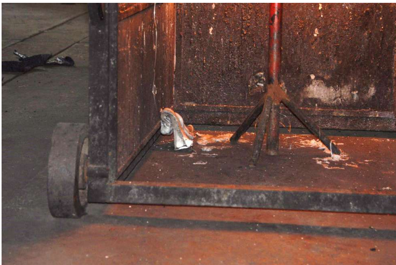
Figure 3.6: Molten debris around the fire source
