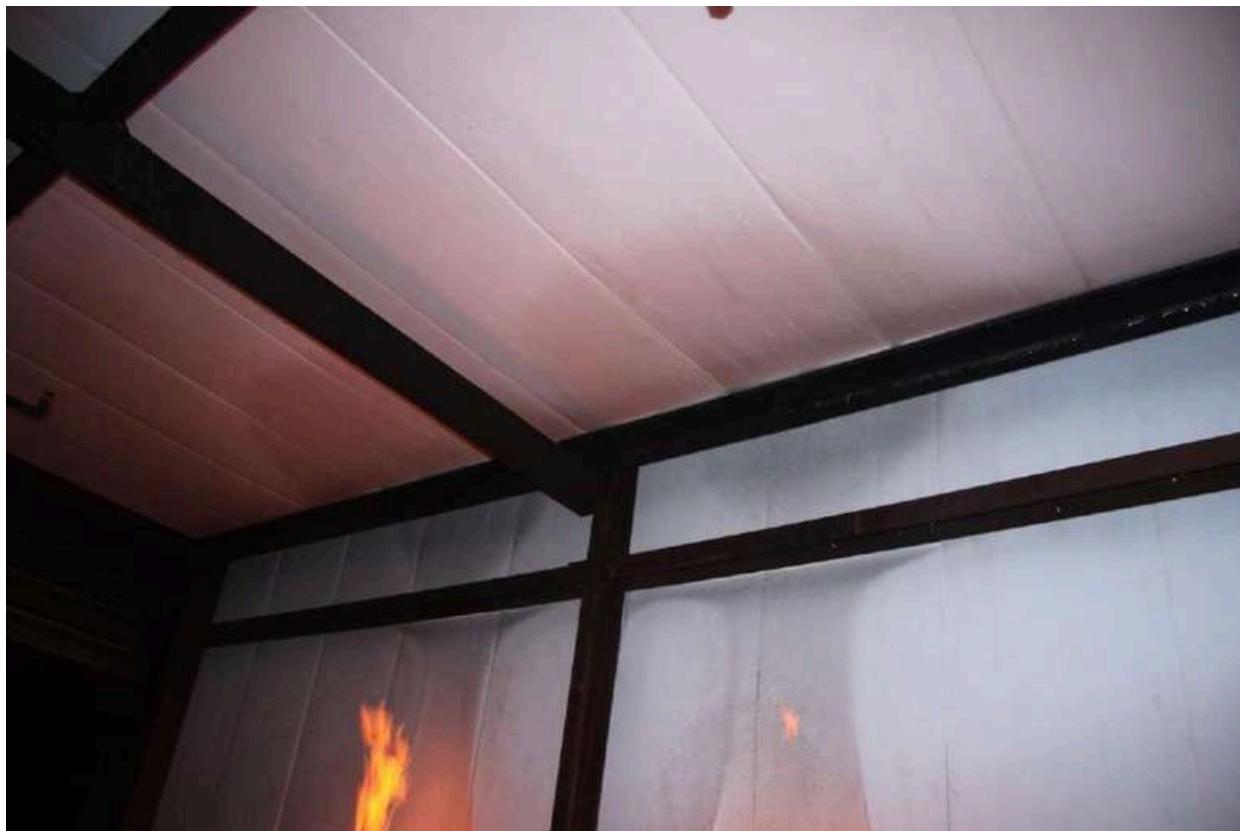
Figure 4.4.6: Heat damage visible on horizontally installed material
